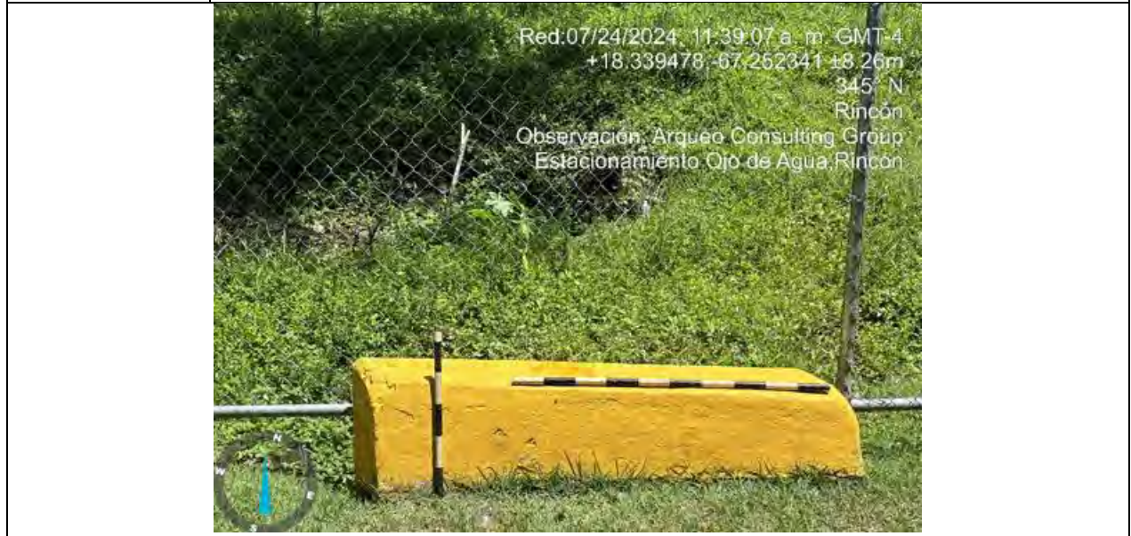
Photo #: 6 Description (North): Concrete drainage system located at the limit of the Residential Santa Rosa and the lot to be developed, near the basketball court. South to north vantage point. Date: 7/24/24
