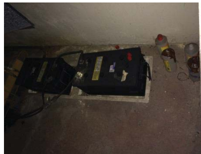
Batteries in Emergency Generator's Room
