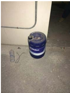
Pail of motor Emergency Generator's Room
