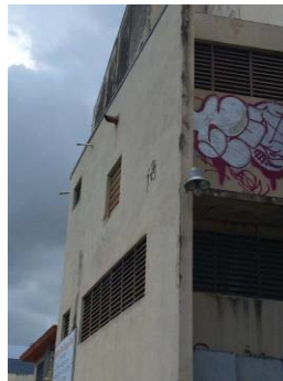
View Emergency Generator's exhaust pipe
