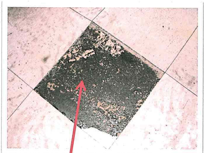
Vinyl Floor Tiles and black mastic NEGATIVE to asbestos
