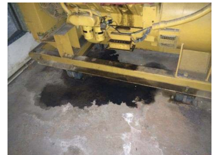
Oil stain in Emergency Generator's Room
