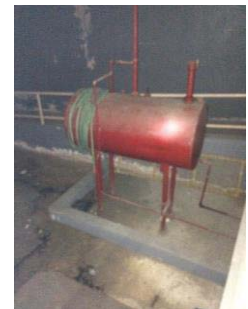
Diesel Tank and Dike
