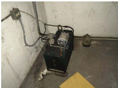
Motor and unidentified container in Emergency Generator's room
