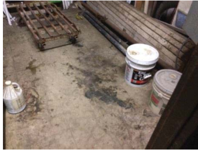
Pails of paint and unidentified liquids, and building materials in a room inside the Building
