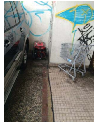
View of the Western Boundary and Electric Generator used in the Café
