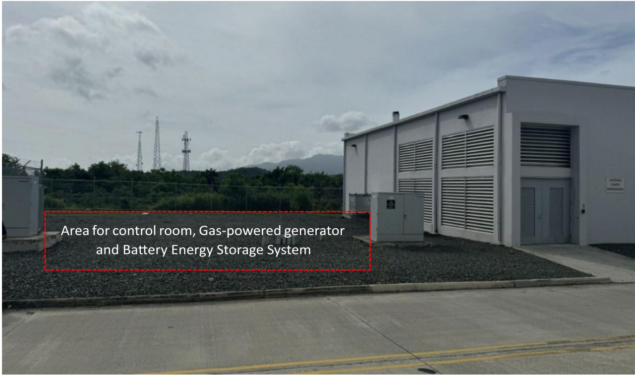
Ground-level photo showing the area next to the building where the existing emergency-power generator units are located and where new equipment will be located.
