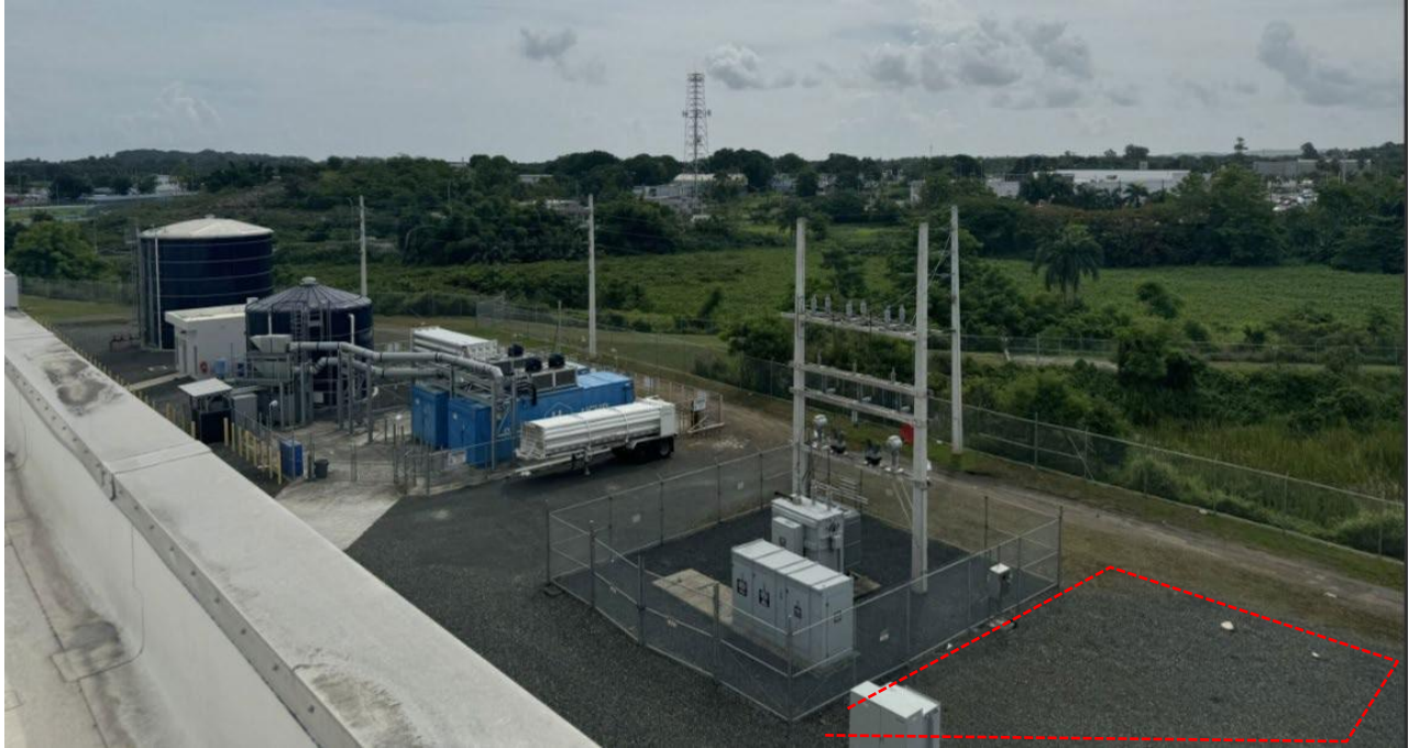
Utilities area showing area where the new equipment and control room will be located.
