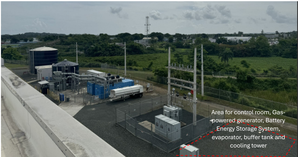
Utilities area showing area where the new equipment and control room will be located.
