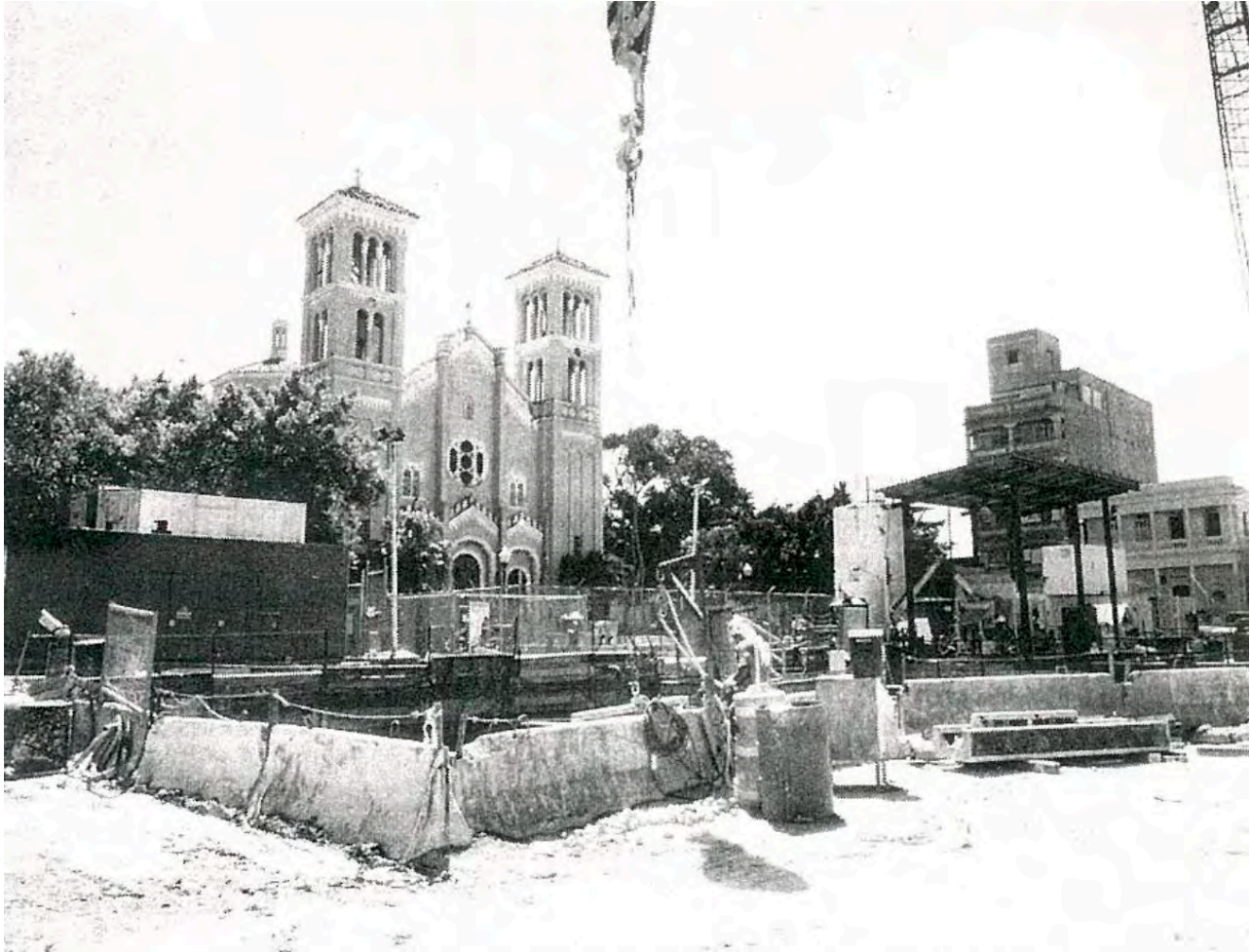
Figure 32. Excavation and filling along the west side of Plaza del Pilar and Ponce de León Avenue during the construction of an underground train tunnel for the Tren Urbano ( ¡Qué huevo! Error en túnel del Tren, Primera Hora, Nydia Bauzá 1999 ).
