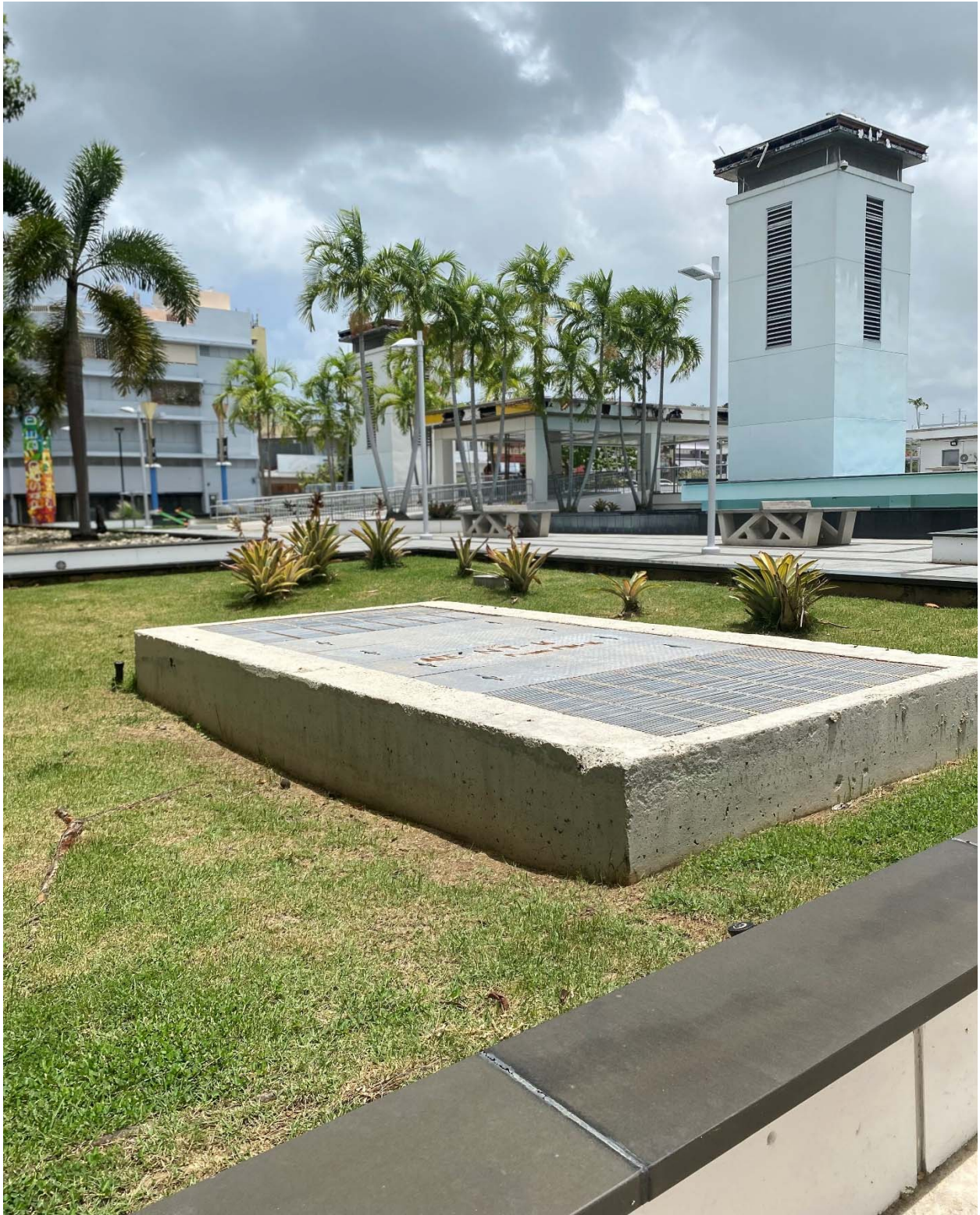
6a: Underground parking ventilation system
