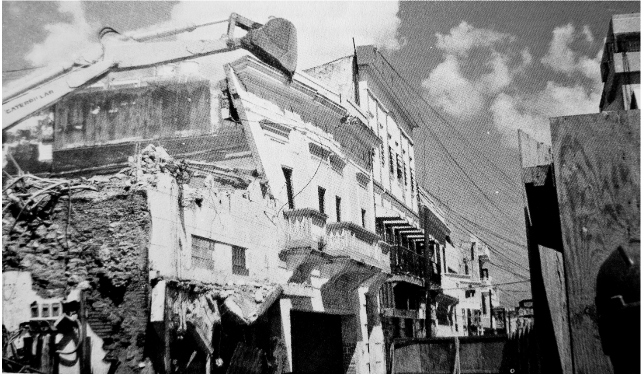
Figure 31. Demolition of three historic buildings in front of Plaza del Pilar for the construction of the Río Piedras section of the Tren Urbano in 1999 (IV Encuentro de Investigadores, Instituto de Cultura Puertorriqueña, 2002:100).
