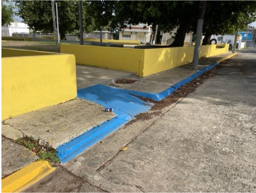
Area 1- Blue Concrete Handicap Ramp & Curb with Lead Based Paint
