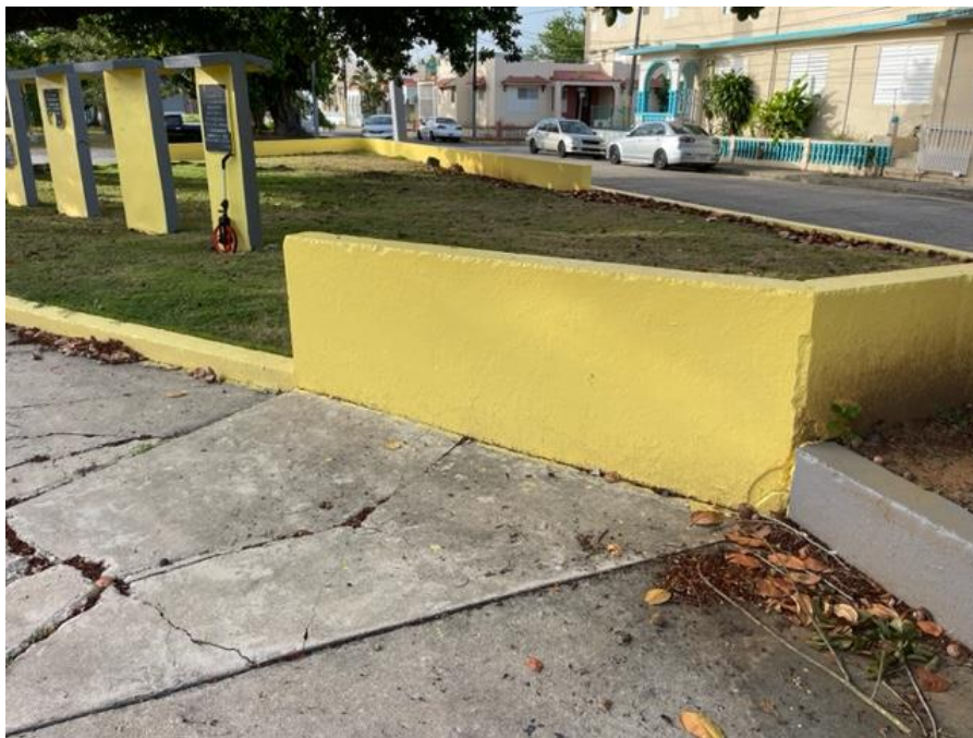
Area 1- Concrete Barriers with Lead Based Paint
