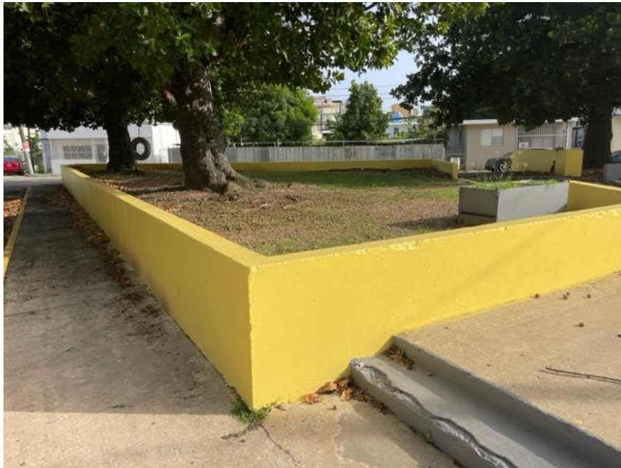
Area 3- Concrete Barriers with Lead Based Paint
