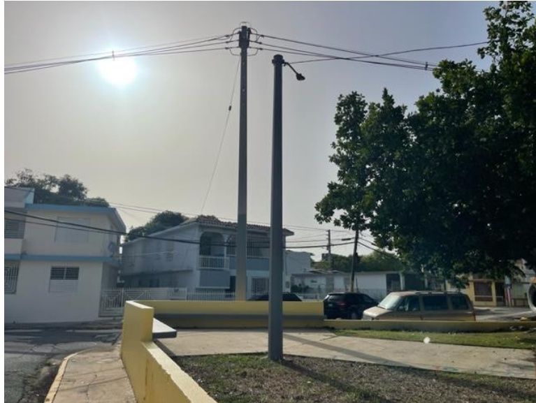
Area 2- Metal Light Post in Center area with Lead Based Paint
