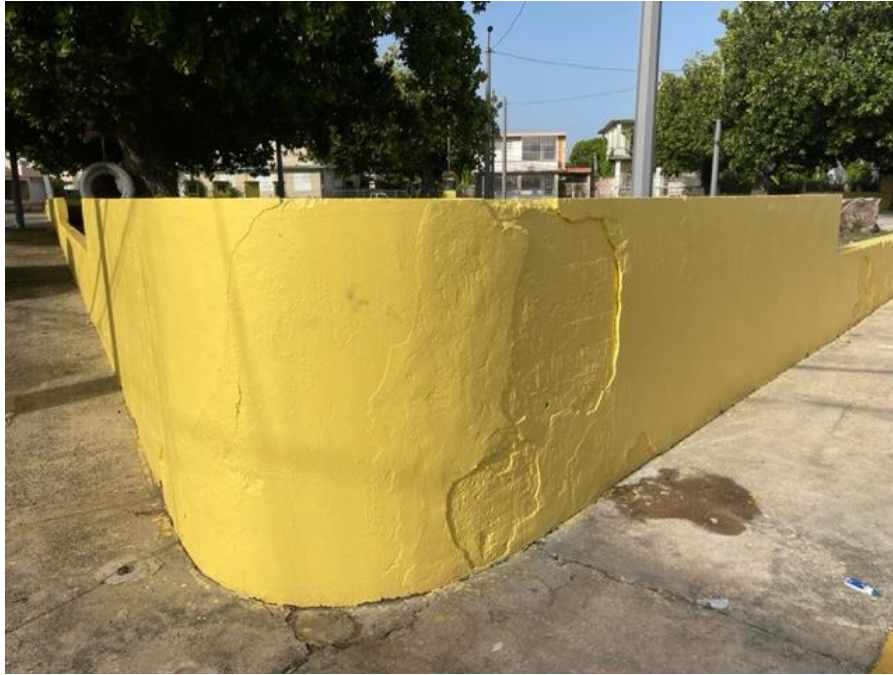
Area 2- Concrete Barriers with Lead Based Paint
