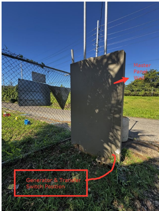
[Electrical Wiring from Master Panel to Generator and Transfer Switch]
