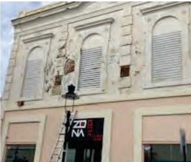
Cream Concrete Wall A, Window Frames, Wall Designs, Upper Trim, Window Upper Trim and Upper Name Area Painted with LBP Exterior Wall A- 2nd Floor, Building #10
