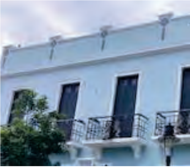
Blue Concrete Wall A, White Concrete Middle Trim and White Concrete Door Frames Painted with LBP Exterior Wall A- 2nd Floor, Building #4
