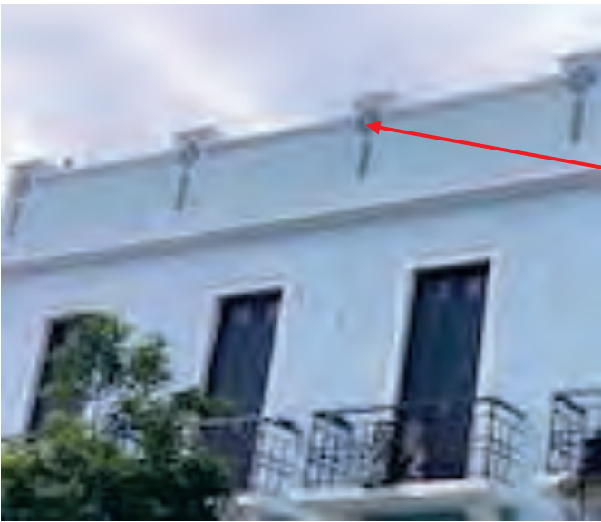
Multicolor Ceramic Mosaics Painted with LBP Exterior Wall A- 2nd Floor, Building #4
