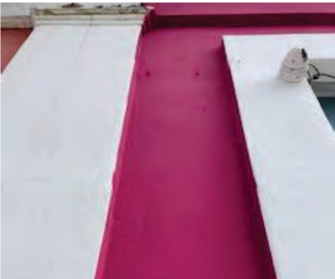
Pink/White Concrete Wall and Column Painted with LBP Exterior Wall A, Building #27
