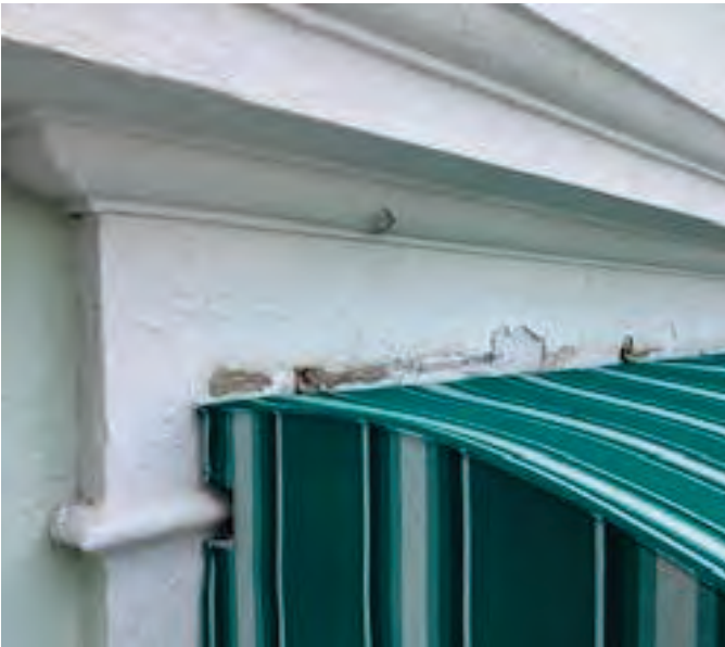
White Concrete Upper Window Frame Painted with LBP Exterior Wall A-B, Building #9
