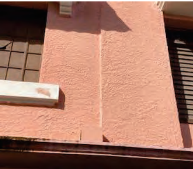
Pink Concrete Wall A Painted with LBP Exterior Wall A- 2nd Floor, Building #17
