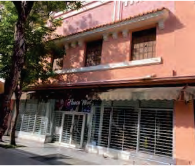
Pink Concrete Wall and Columns Painted with LBP Exterior Wall A- 3rd Floor, Building #17
