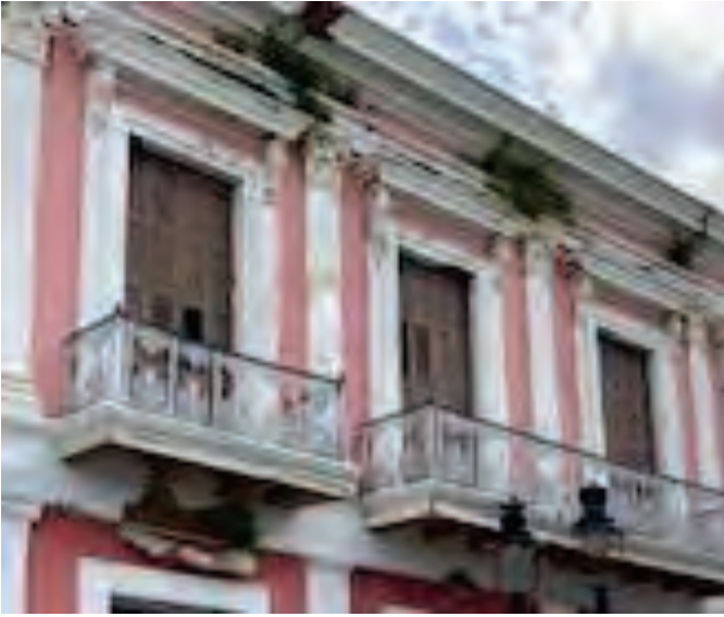
Brown Metal Handrail, Pink Concrete Wall, White Concrete Columns, Door/Window Frames and Trim Painted with LBP Exterior Wall A- 2nd Floor, Building #28
