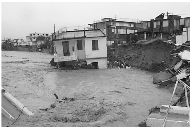
House damaged by floodwaters from the Río Viví in downtown Utuado, Puerto Rico. Photograph by Heriberto Torres-Sierra, September 1998, USGS.
