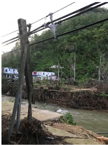
Source: NYPA/Con Edison Damage Assessments
