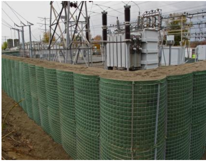
Flood Barrier Source: Con Edison
