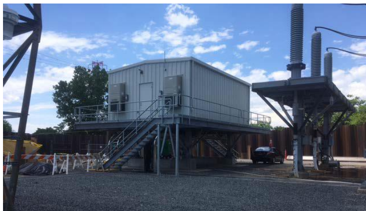
Modular Control Building
