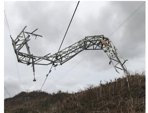
Source: NYPA/Con Edison Damage Assessments
