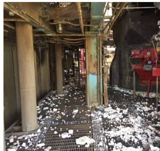
Source: NYPA/Con Edison Damage Assessments
