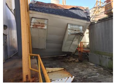
Source: NYPA/Con Edison Damage Assessments
