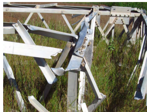
FIGURE 7. Detail of damage in a transmission tower with fractured braces. (Photo: A. Kwasinski).
