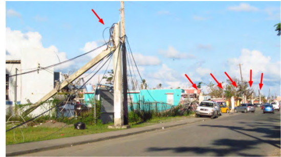
FIGURE 5. Multiple broken concrete poles in Punta Santiago. (Photo: A. Kwasinski).
