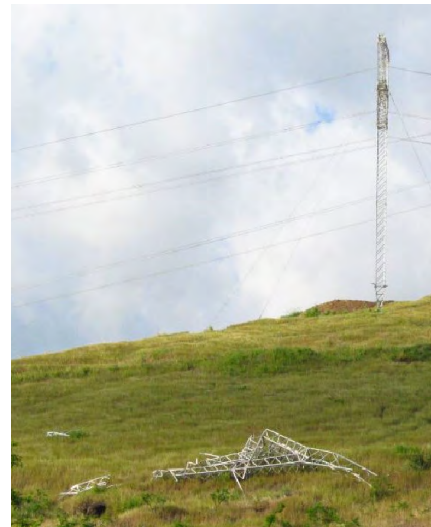
FIGURE 6. One of the many fallen transmission towers in Puerto Rico. (Photo: A. Kwasinski).
