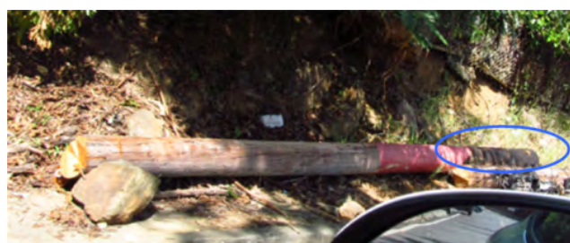
FIGURE 9. A 30 ft long fallen pole with an oval showing its buried portion. This buried portion measured approximately 3.7 ft., which is less than the 5 ft. 6 in. used in a utility in Florida [22]. (Photo: A. Kwasinski).
