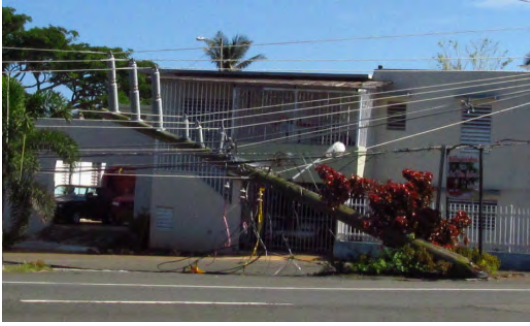
FIGURE 4. A fallen transmission wooden pole. (Photo: A. Kwasinski).
