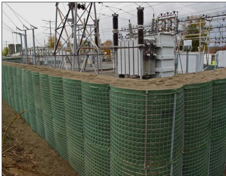
Figure 4-6. Substation Flood Barrier
