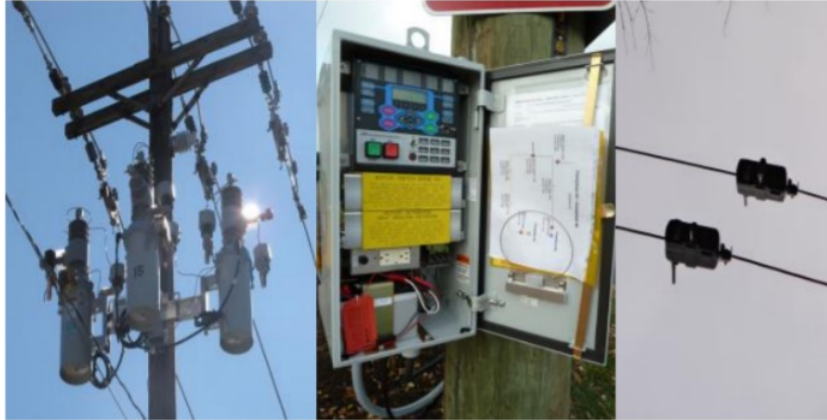
Figure 4-8. Electronic Reclosers, Control Units and Line Sensors Installed by Duke Energy
