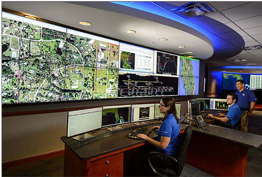
Figure 5-6. Modern Control Center
