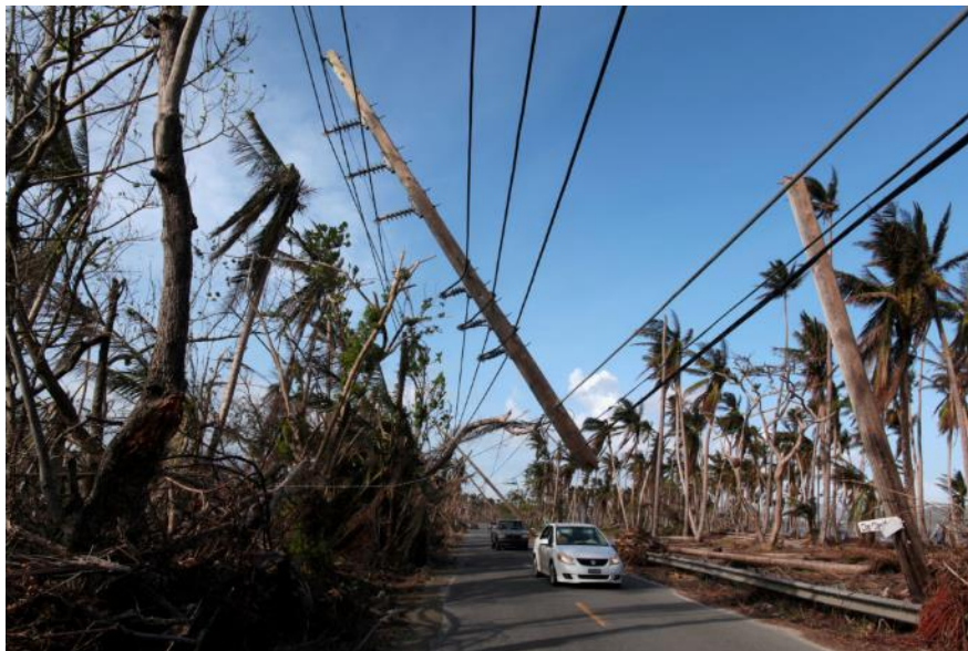
Figure 1. Broken Distribution Poles After the Storm
