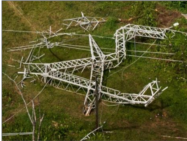
Figure 2-5. Transmission Structure Knocked Down by Hurricane Maria
