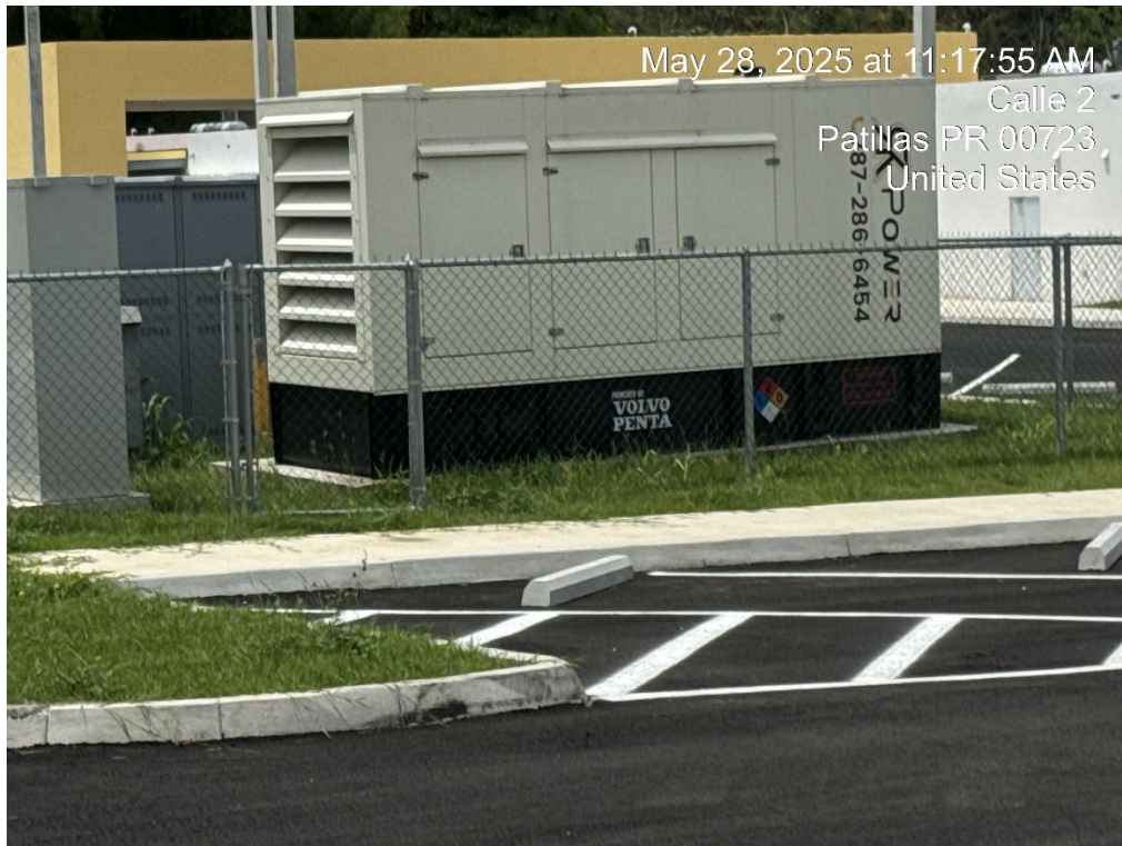
School, distance 984 ft, 500-gal diesel
