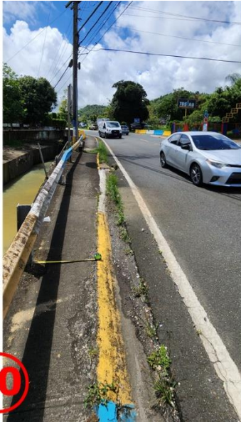
Photo location # 10- Existing sidewalks showing no ADA compliance width.
