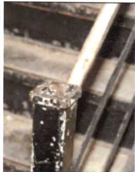
FIGURE 12.5 A metal railing before abatement.
