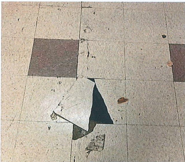
Asbestos Containing Black Mastic under Pink and Cream Vinyl Floor Tiles Administration Area
