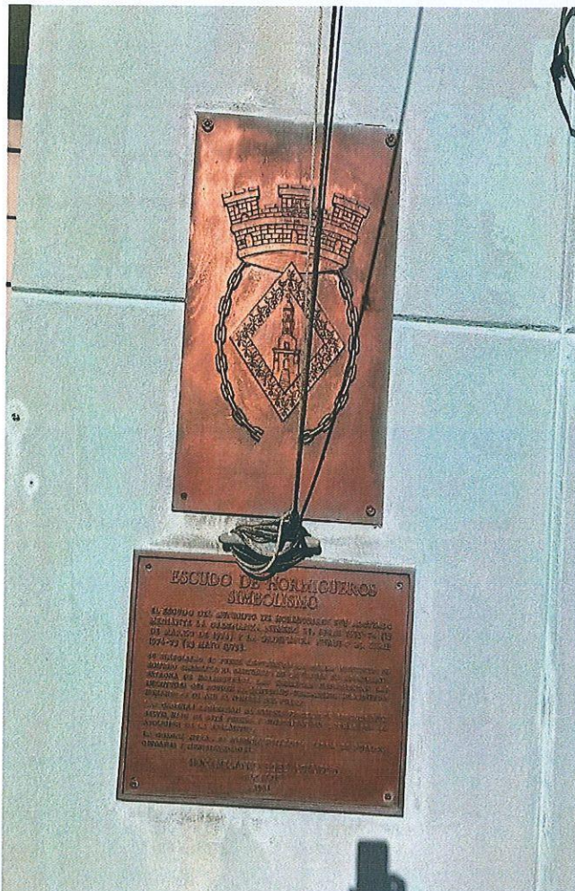
Brown Metal Commemorative Plaque Painted with LBP Exterior of Structure
