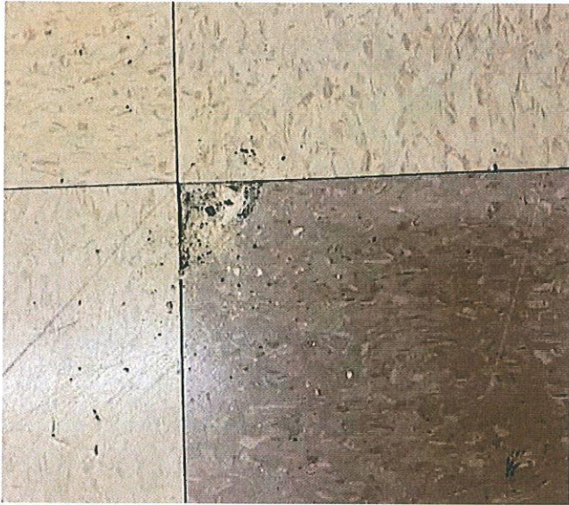
Asbestos Containing Black Mastic under Pink and Cream Vinyl Floor Tiles Auditorium Area
