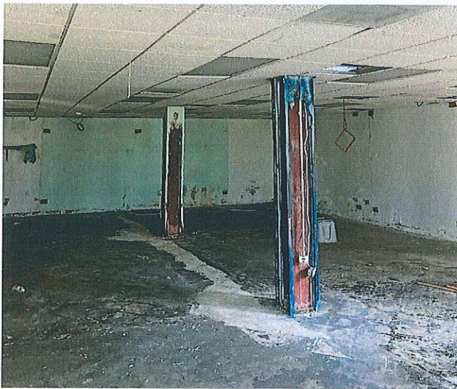
Asbestos Containing Black Mastic on Floor Room 201- Basement
