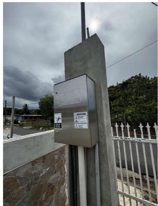
New Transfer Switch
