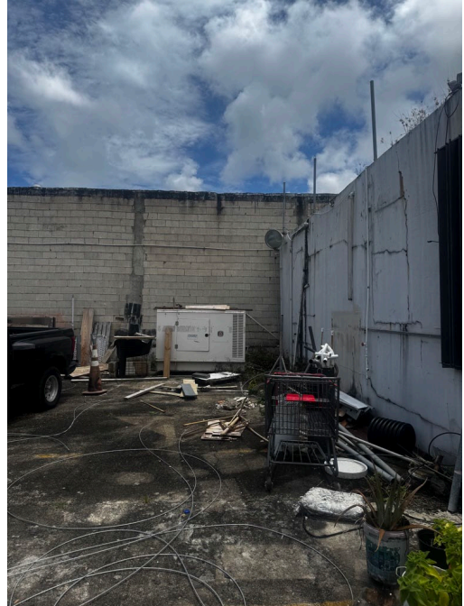
AST | This generator belongs to neighbor's property | Located at Rear of the property
