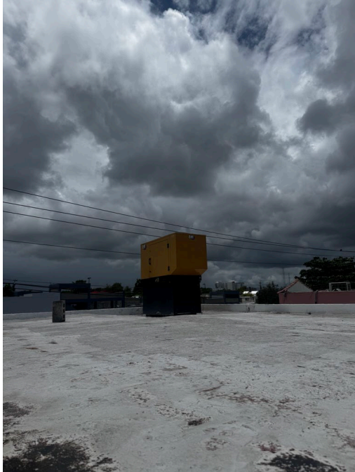
AST | New Generator
